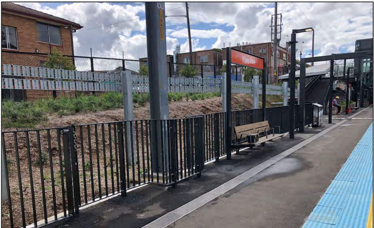
Photo 4. General current condition of Platform 1, Wiley Park Station. Date: 21 April 2023.
