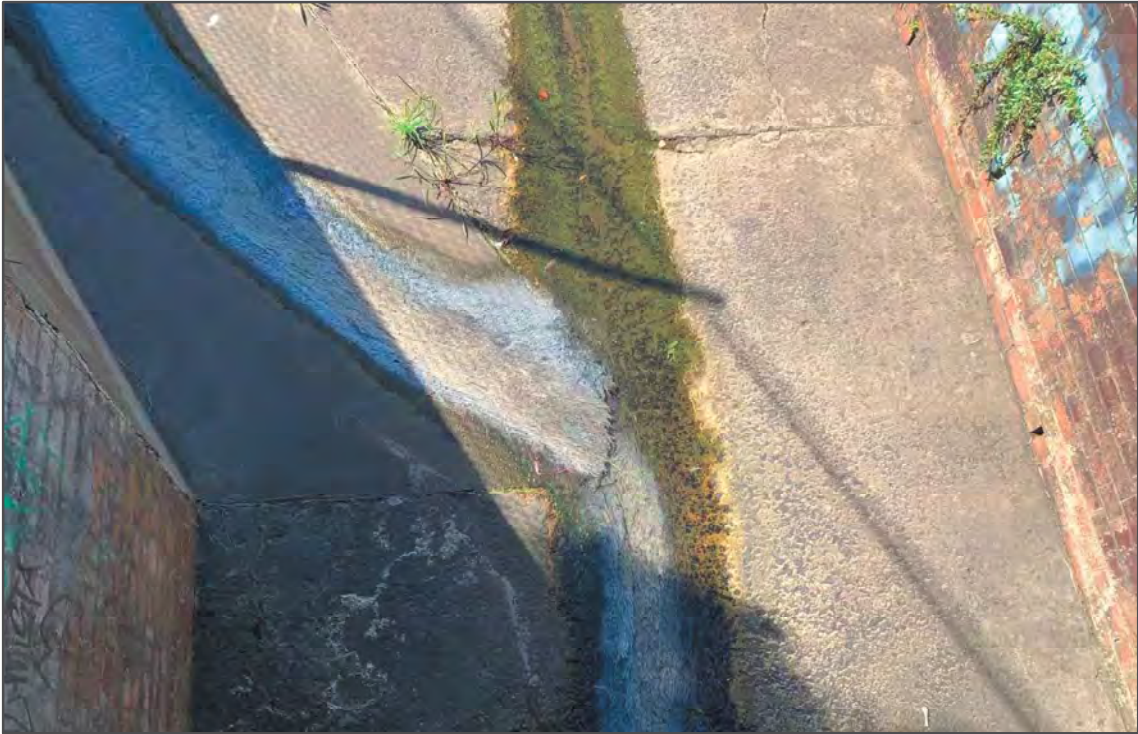
Photograph 2. Condition observed from sampling location of WP1 during the monitoring event – 6 December 2023.
