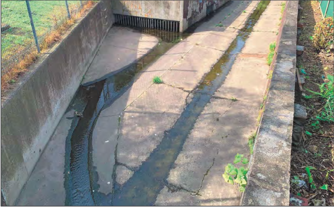
Photograph 1. Condition observed from sampling location of WP1 during the monitoring event – 15 September 2023.
