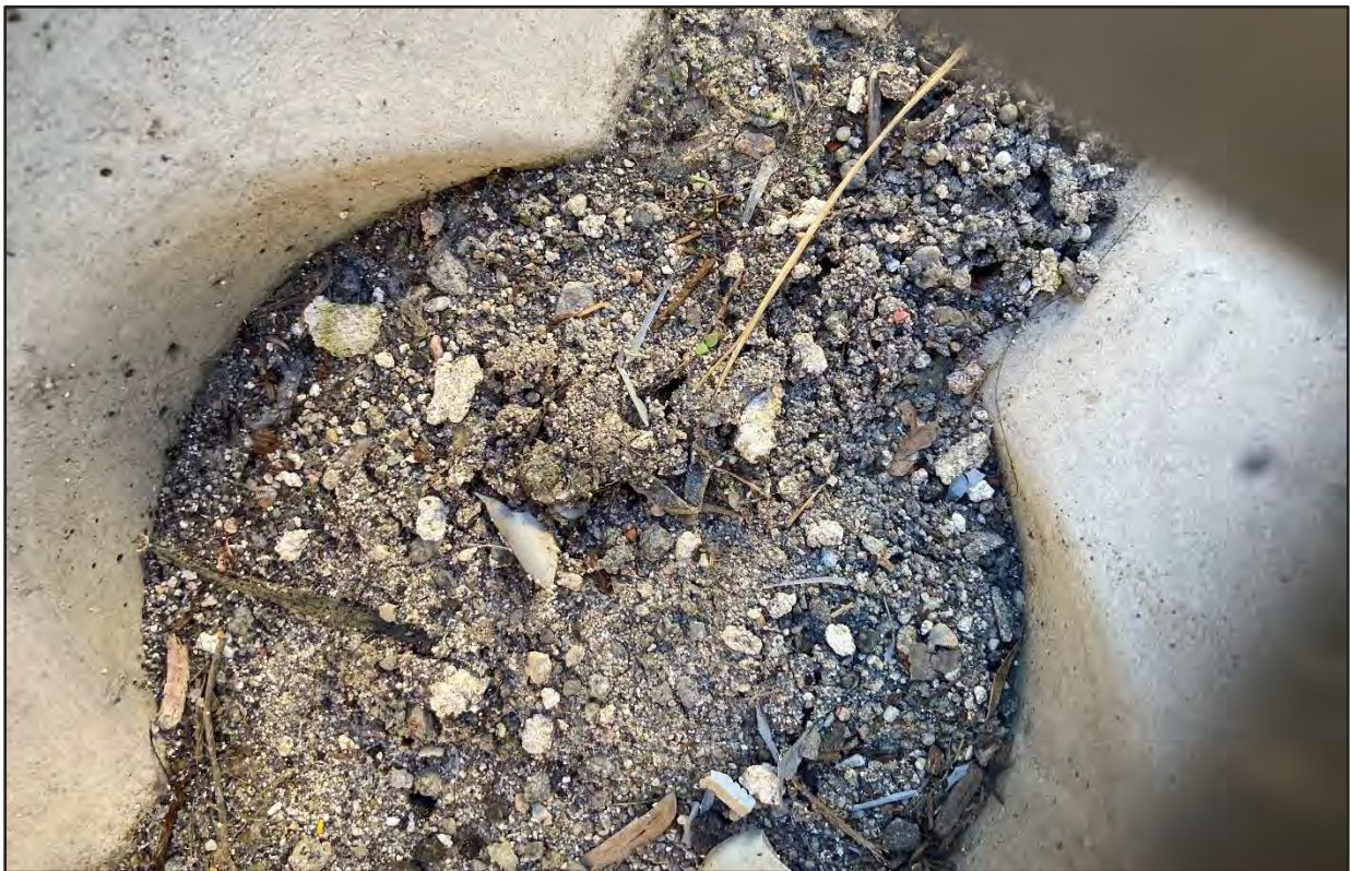
Photo 2. Aco drain condition prior to the sediment removal on 17 March 2023.
