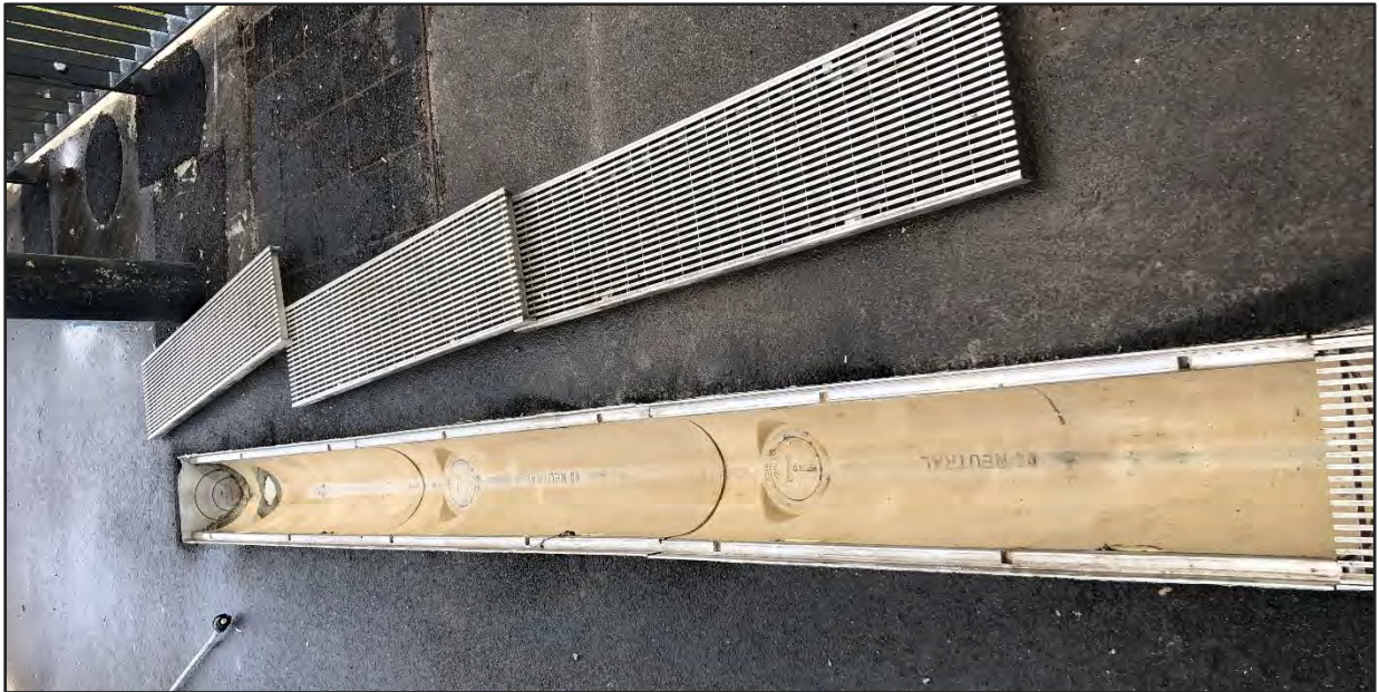
Photo 3. Aco drain condition after the sediment removal on 21 April 2023.
