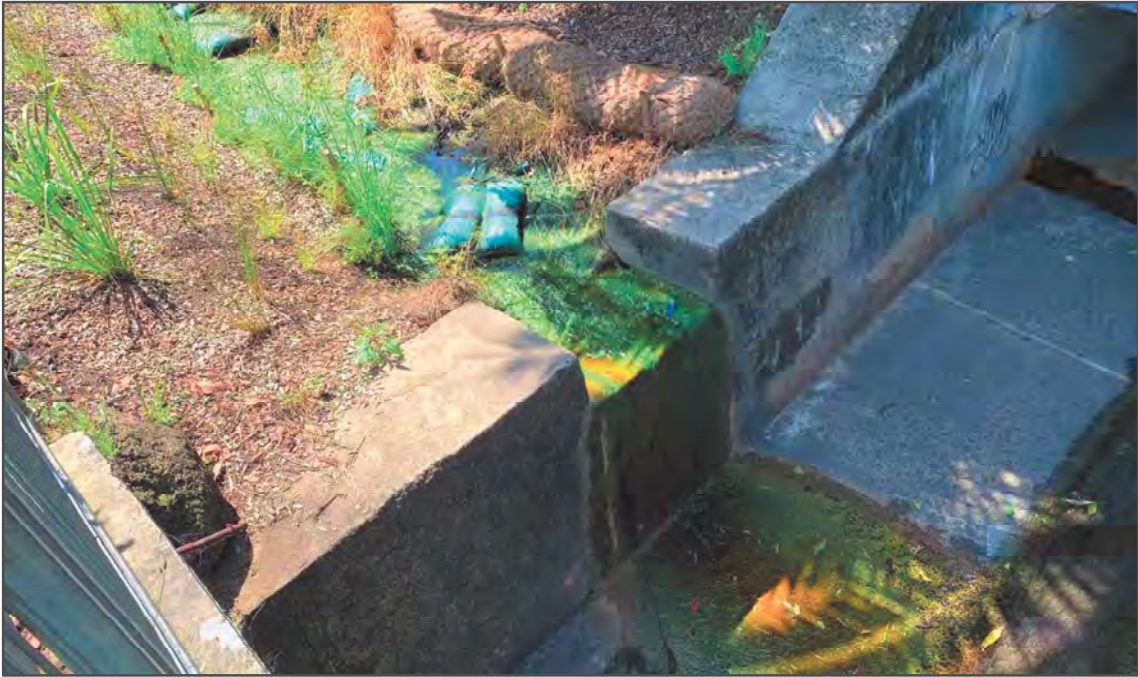
Photograph 4. Condition observed from downstream discharge point WP2-DP1 that was located within the rail corridor and immediately upstream / south from WP2 during the monitoring event. Significant algae growth was observed at this location at the time of monitoring – 6 December 2023.
