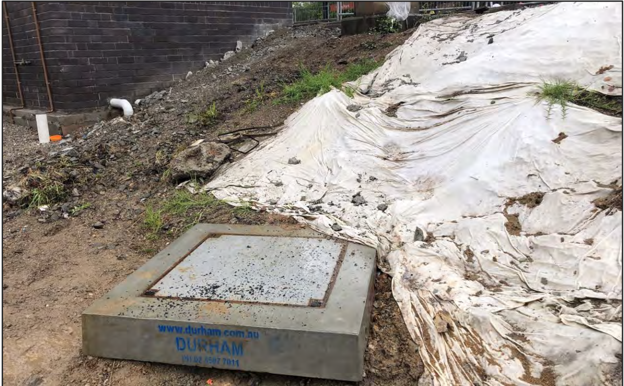
Photo 6. No access was obtained for the two drainage pits located between the downstream (south-western) end of the aco drain and the downstream discharge headwall for inspection and validation test. Date: 5 October 2022.
