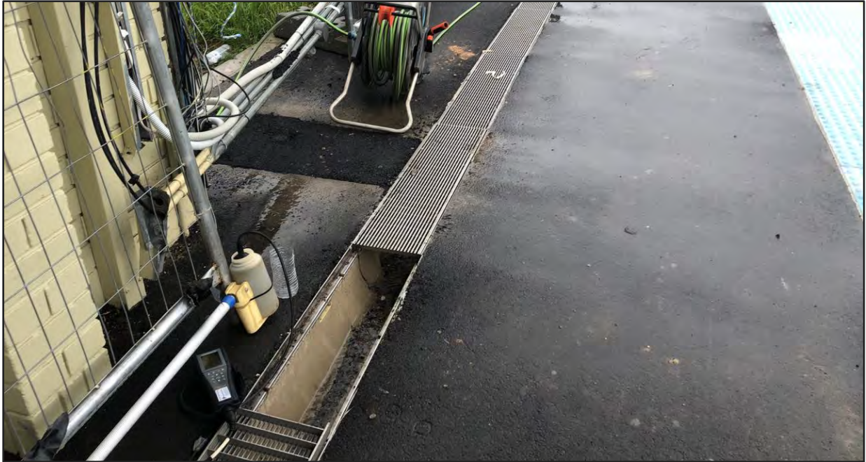
Photo 1. Aco drain condition prior to the sediment removal on 5 October 2022.
